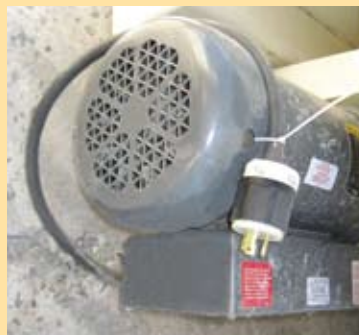
Auxiliary 5-hp motor can be powered by a small generator in emergencies.
